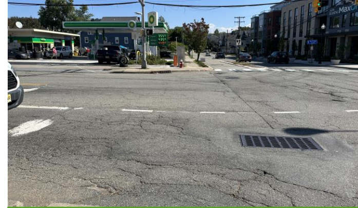
Missing crosswalk for Ridgedale Avenue approach
