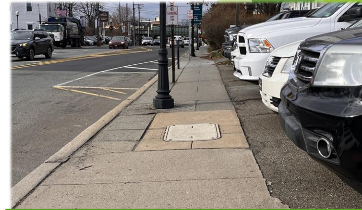
Non-compliant sidewalks immediately adjacent to private parking area in northwest corner
